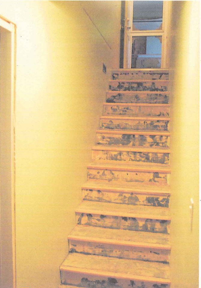
LOOKING UP STAIRWAY STAIRS FROM INTERIOR SUITE DOOR UP TO EXT DOOR TO CARPORT.
